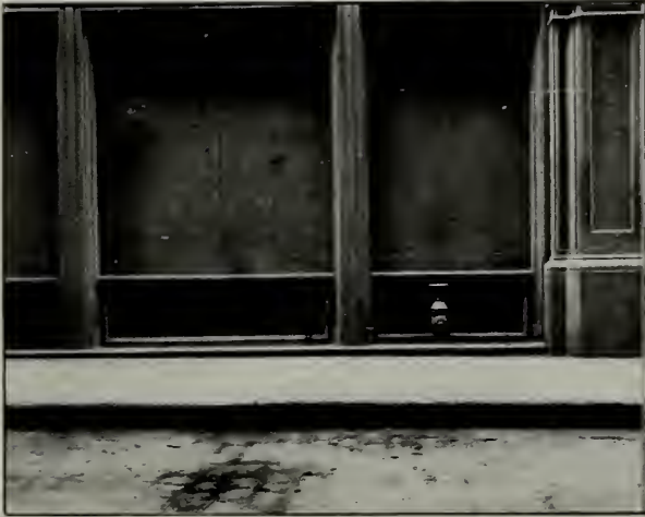
FIG. 1.— UNSCREENED BASEMENT VENTILATOR.
