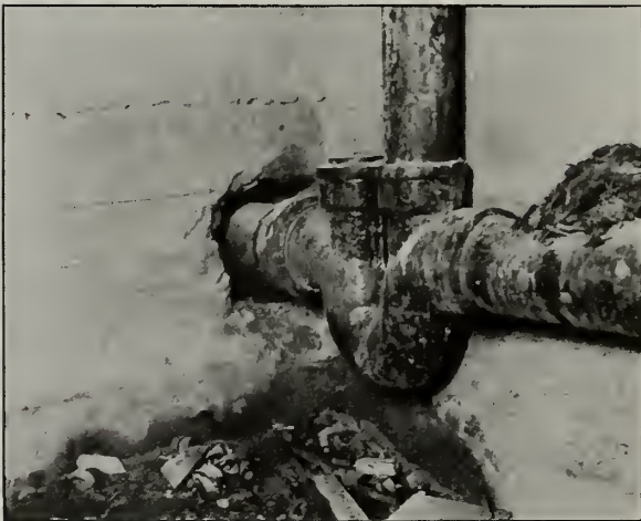
FIG. 2.—DEFECTIVE BASEMENT WALL (OPENING MADE FOR THE INSTALLATION OF HOUSE SEWAGE SYSTEM).
