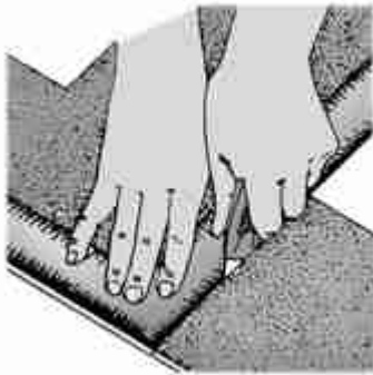
FIG. 3 - Plastic laminate can be cut with a utility knife or using special laminate blades.
