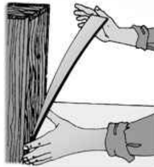
FIG. 10 - Sheets applied to vertical areas do not normally require a protective shield of paper.
