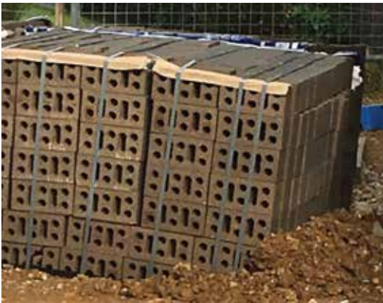
Figure 9 – Example of poor brick storage
