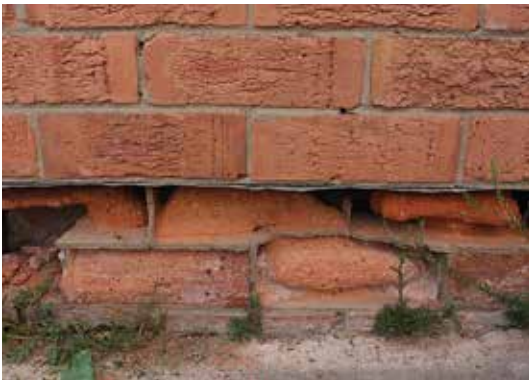
Figure 1 – Salt attack damage to masonry unit
