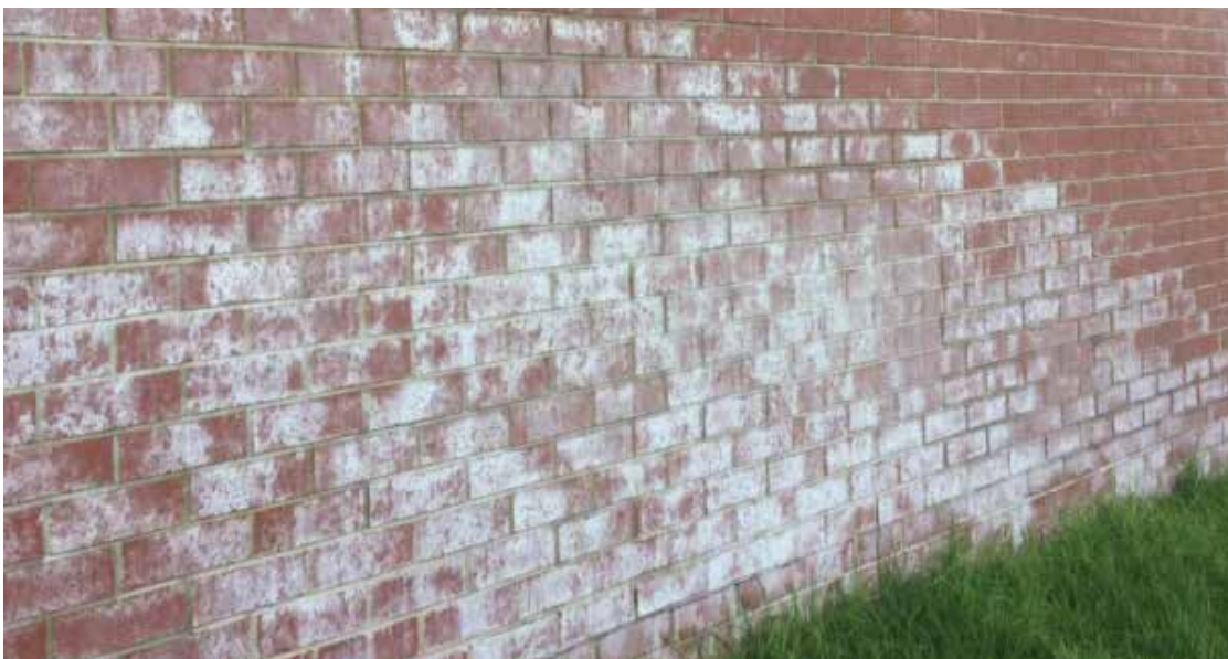
Figure 3 – Efflorescence on brickwork
