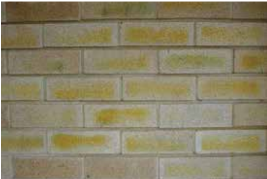
Figure 7 – Vanadium staining on brick face
