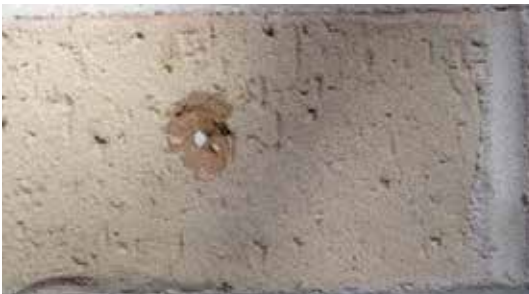
Figure 5 – Lime pitting appearing on the face of the brick
