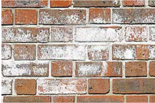
Figure 4 – Insoluble white deposits on brickwork
