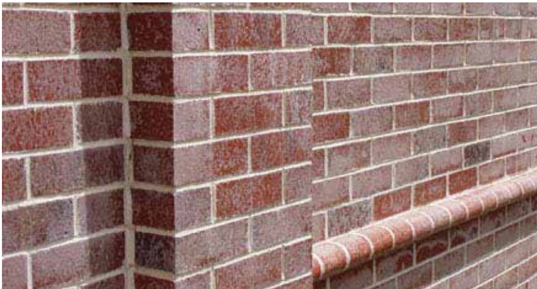
Figure 4 – Brickwork effected by efflorescence
