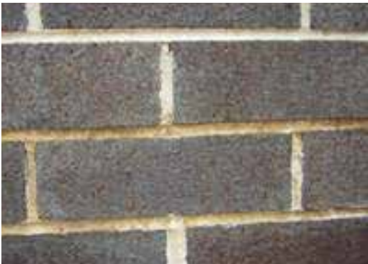
Figure 6 – Iron Staining in Mortar Joints
