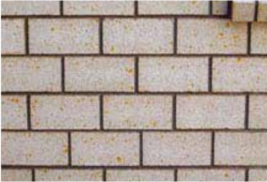
Figure 5 – Iron Staining on Brick Faces
