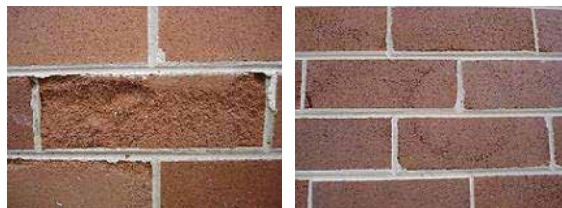
Figure 1 – Dry press brick damage due to high pressure cleaning
