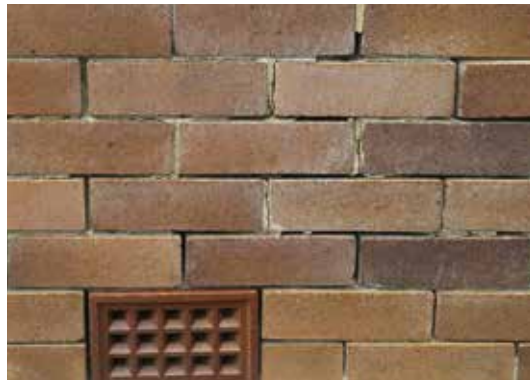
Figure 2 – Salt attack damage to mortar
