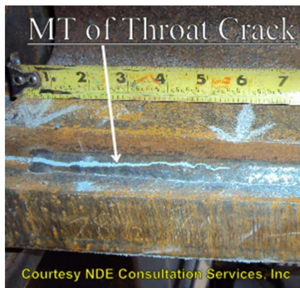
Figure 20: MT of throat crack
