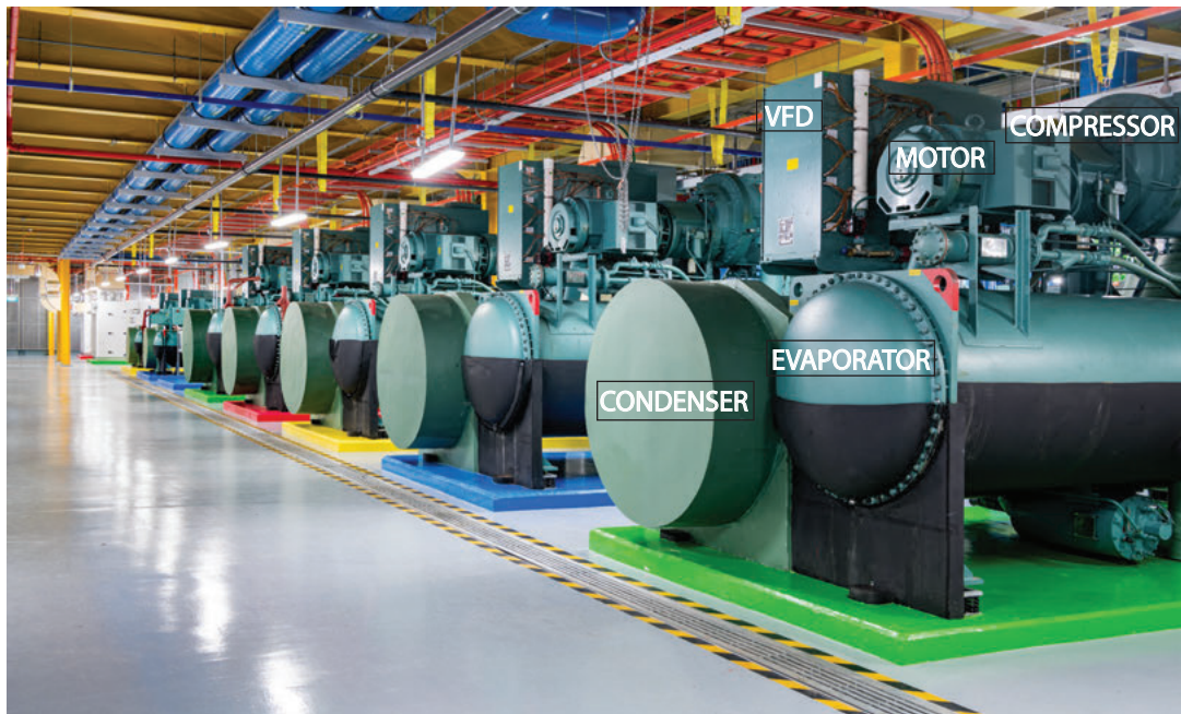
Figure 4.11: Water-cooled centrifugal chiller.
