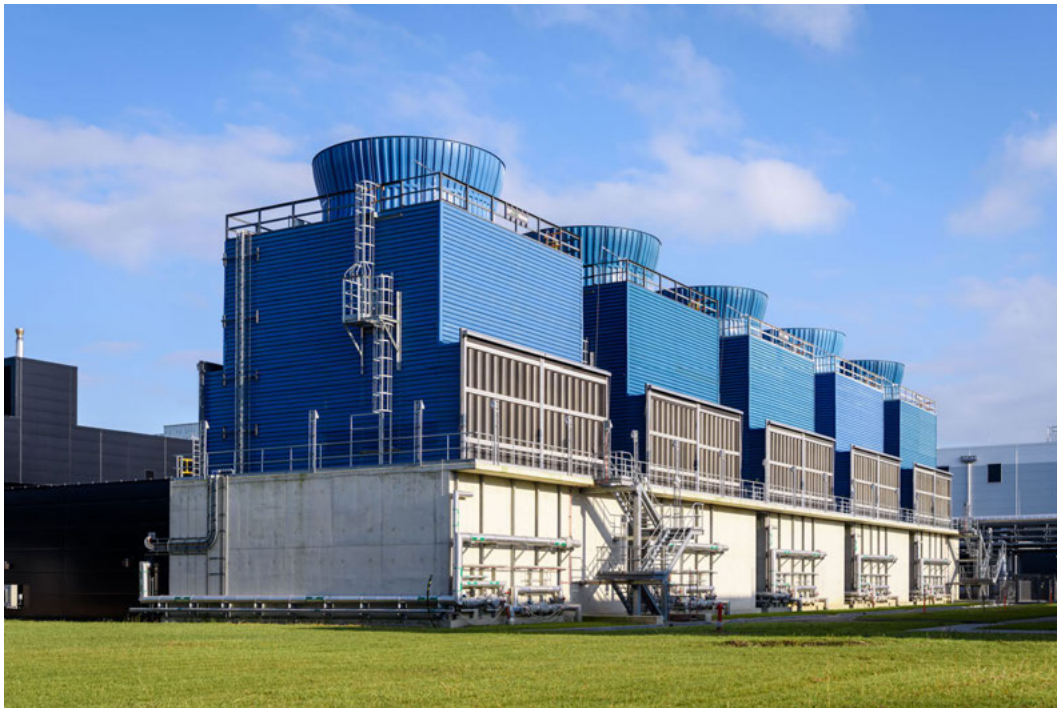
Figure 4.12: Data center cooling towers.
