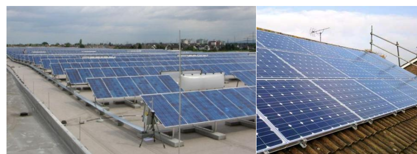
Figure 7-2 PV array on flat and pitched roofs
