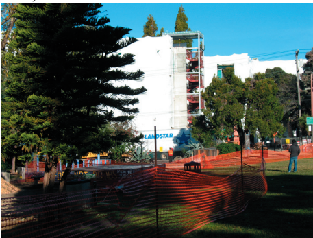
UC ADMINISTRATORS CLAIM that the students who will someday live in this unfinished dorm currently under construction insisted on improving their views by cutting down trees in People's Park.
