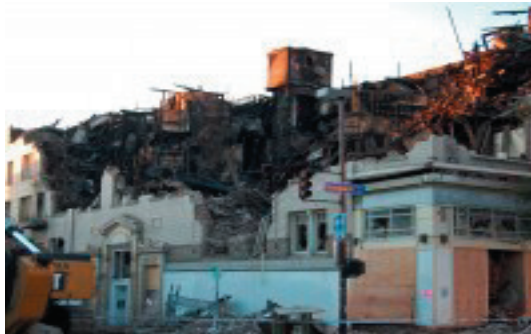
THE FIRE AND DEMOLITION at the corner of Haste and Telegraph had no effect on shoppers, who really enjoy this sort of challenge.
