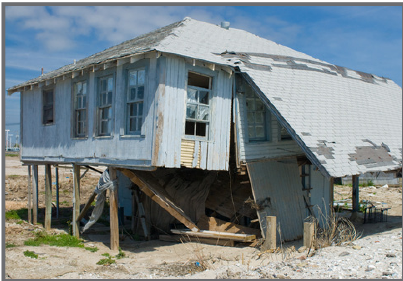
Aftermath of Hurricane Katrina
